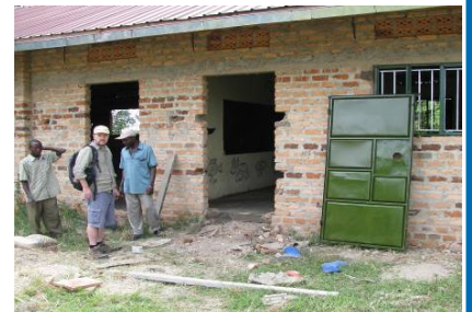
The classroom we kitted out: concrete floor and windows completed, door awaiting fitting at Kiganda School
